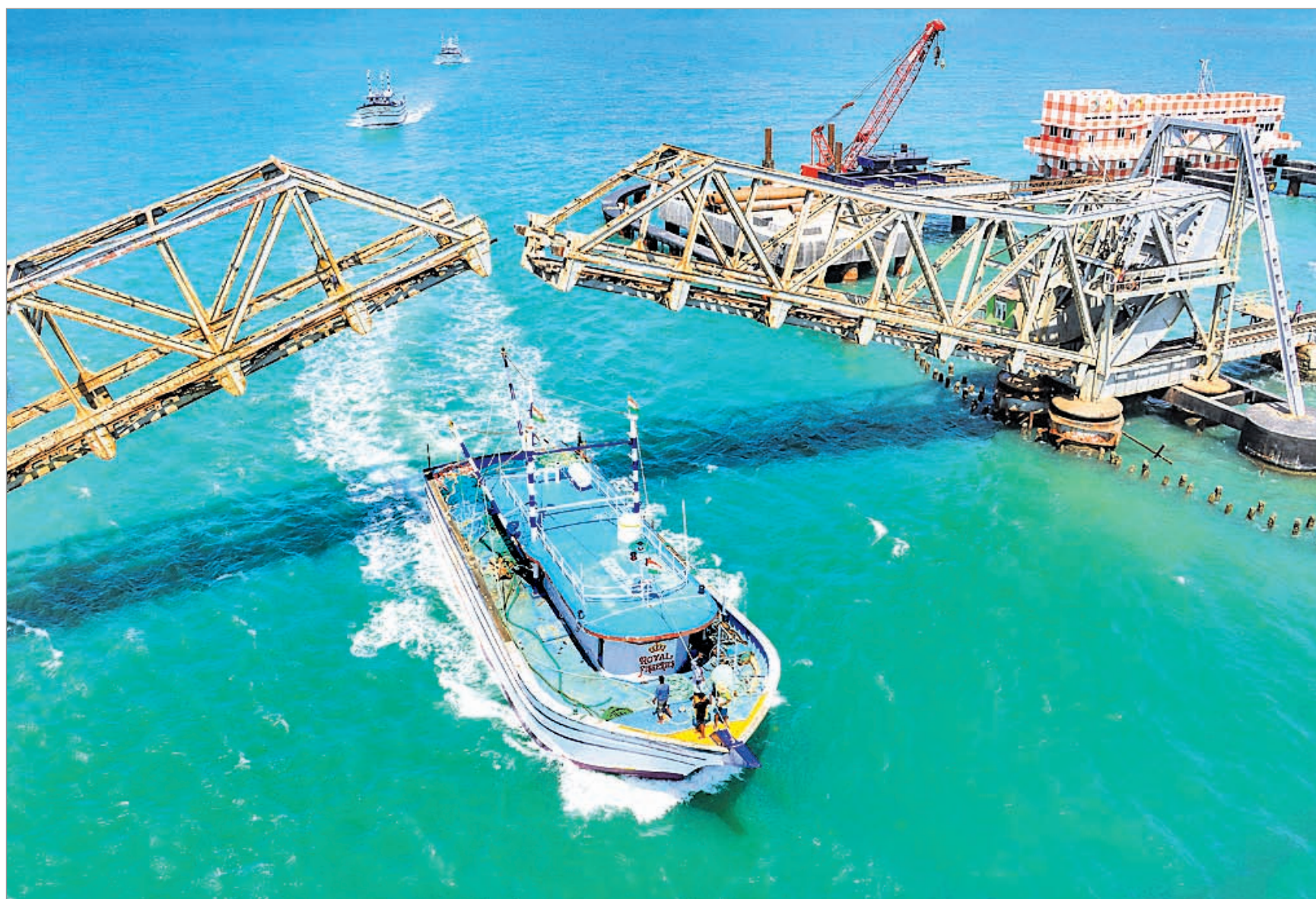
SAFE PASSAGE The suspension railway bridge in Pamban opens for fishing boats in Tamil Nadu's Rameswaram, Thursday
