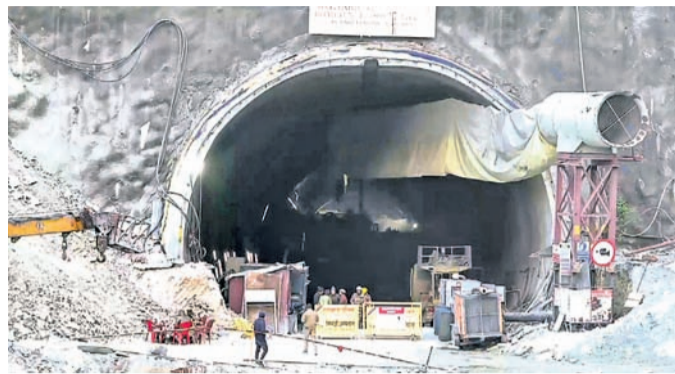
Security personnel at the under-construction tunnel between Silkyara and Dandalgaon on the Brahmakhal-Yamunotri national highway
