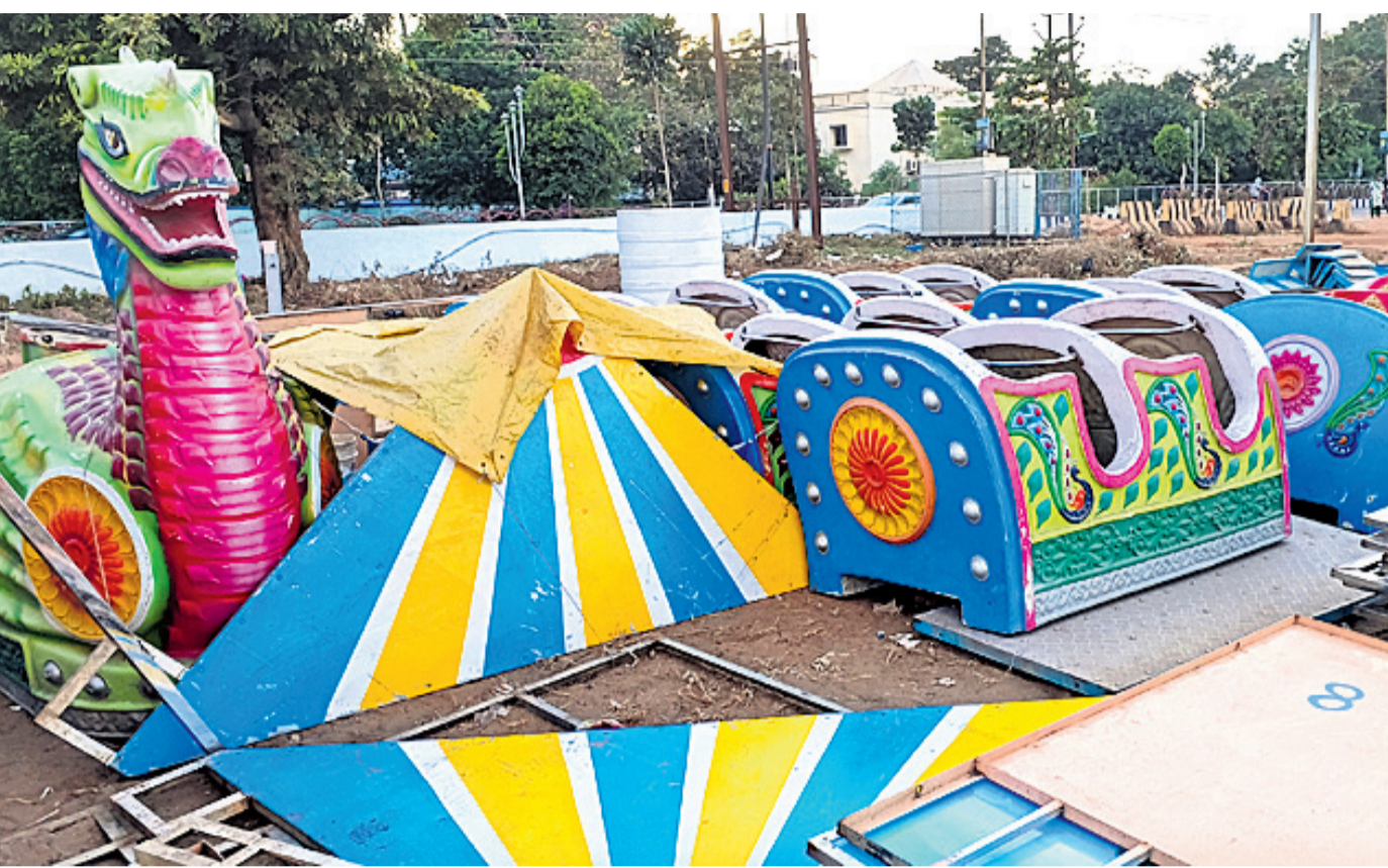
TRADE FAIR AHEAD: Installation of a Ferris wheel in progress at Baliyatra Ground in Cuttack, Friday, as state gears up for the biggest open air trade fair OP PHOTO
