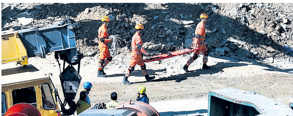
mountain was drilled from the top to about 45 meters to rescue the trapped workers and the debris was still lying in the tunnel, he said.
