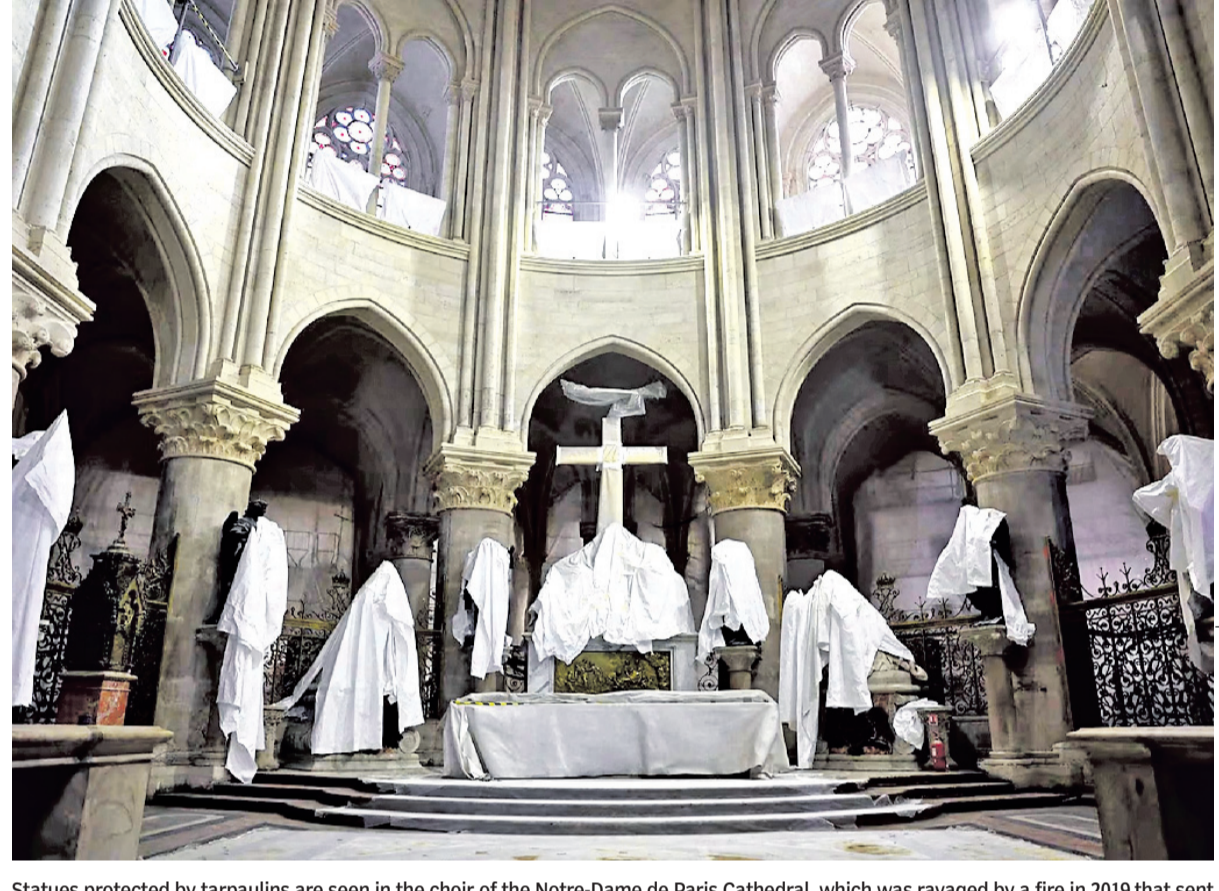
Statues protected by tarpaulins are seen in the choir of the Notre-Dame de Paris Cathedral, which was ravaged by a fire in 2019 that sent its spire crumbling down, as restoration works continue a year before its reopening to the public in Paris, France
