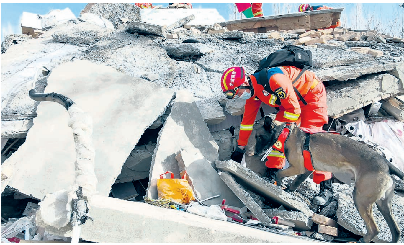
RESCUE OPS: A rescuer uses a sniffer dog to search for survivors at collapsed houses following a massive earthquake in Dahejia Township of Jishishan Bao'an, Dongxiang, Salar Autonomous County in Linxia Hui Autonomous Prefecture, northwest China's Gansu Province, Tuesday. At least 127 people were killed and over 700 others injured when a powerful earthquake of 6.2 magnitude jolted a mountainous region of northwestern China late Monday night, the deadliest in the quake-prone region in nine years. (REPORT ON P10)
