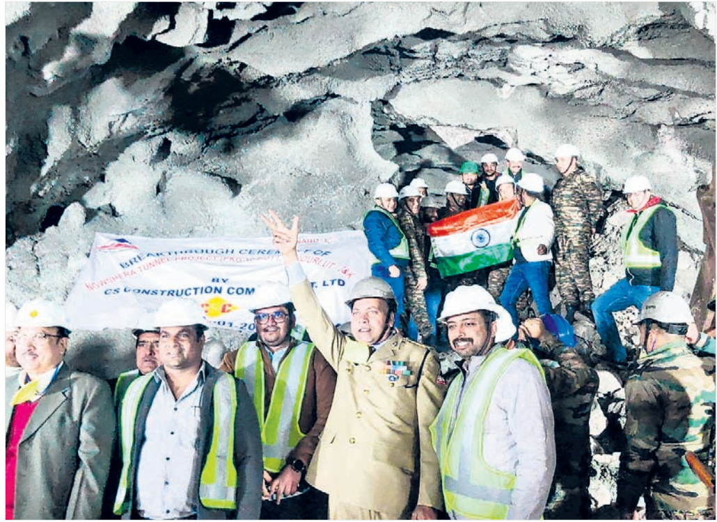
Border Roads Organisation personnel along with engineers and workers during the breakthrough ceremony of Nowshera tunnel project, in Jammu & Kashmir. The tunnel is being constructed on Jammu-Poonch highway
