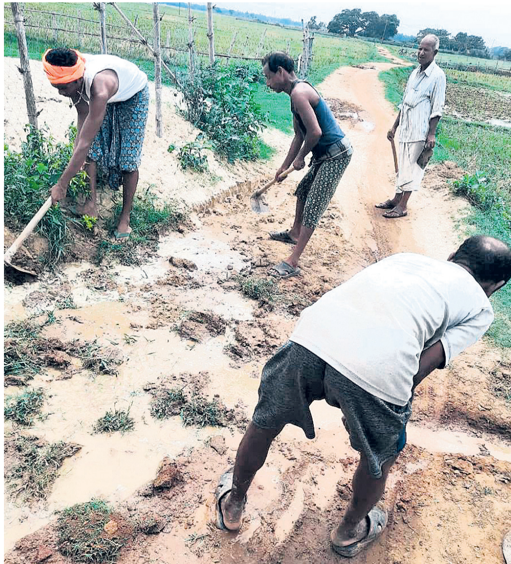
SELF SERVICE: Locals repair the village road connecting Raipur Square to Talagadia in Baniadiha panchayat of Baliaapal block under Balasore district after the administration failed to address their pleas, Wednesday OP PHOTO
