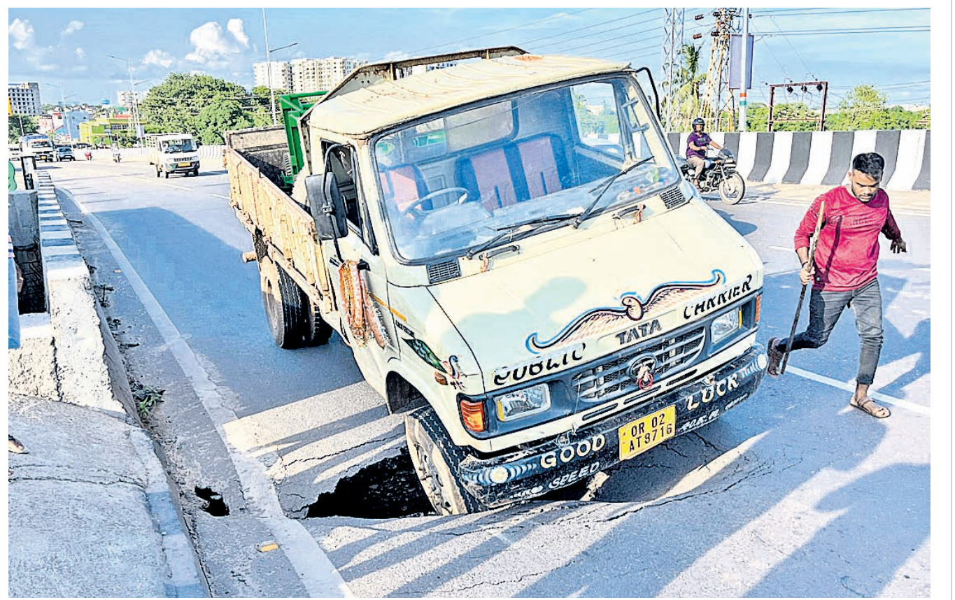
LURKING DANGER: A mini-truck falls into crater after portion of national highway 16 caves in at Dumduma in Bhubaneswar, Monday PIC: MANORANJAN MISHRA
