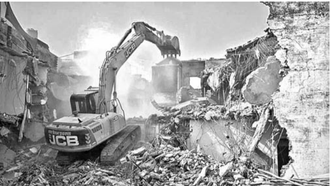
The spate of bulldozing in states like UP, MP, and Delhi, under the cover of the Municipality Act, is an affront to our governance's failure to mete out basic socio-economic justice of decent livelihood, and shelter to all our citizens
