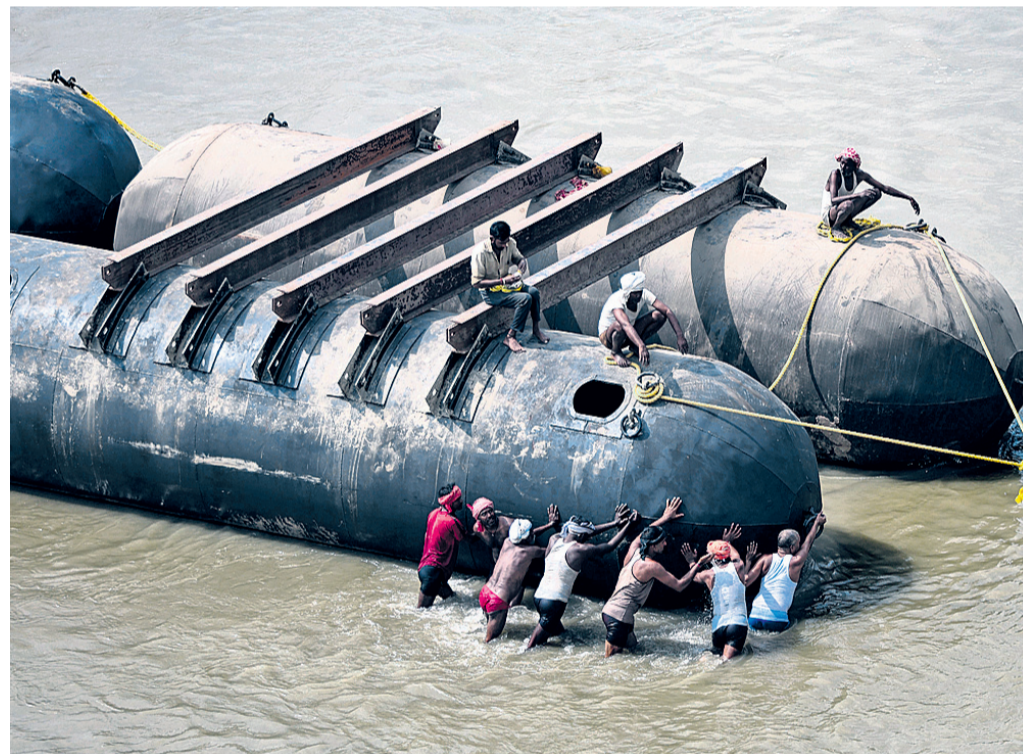
Labourers build a pontoon bridge on the Ganga river during preparations for the upcoming 'Maha Kumbh Mela' festival, in Prayagraj
